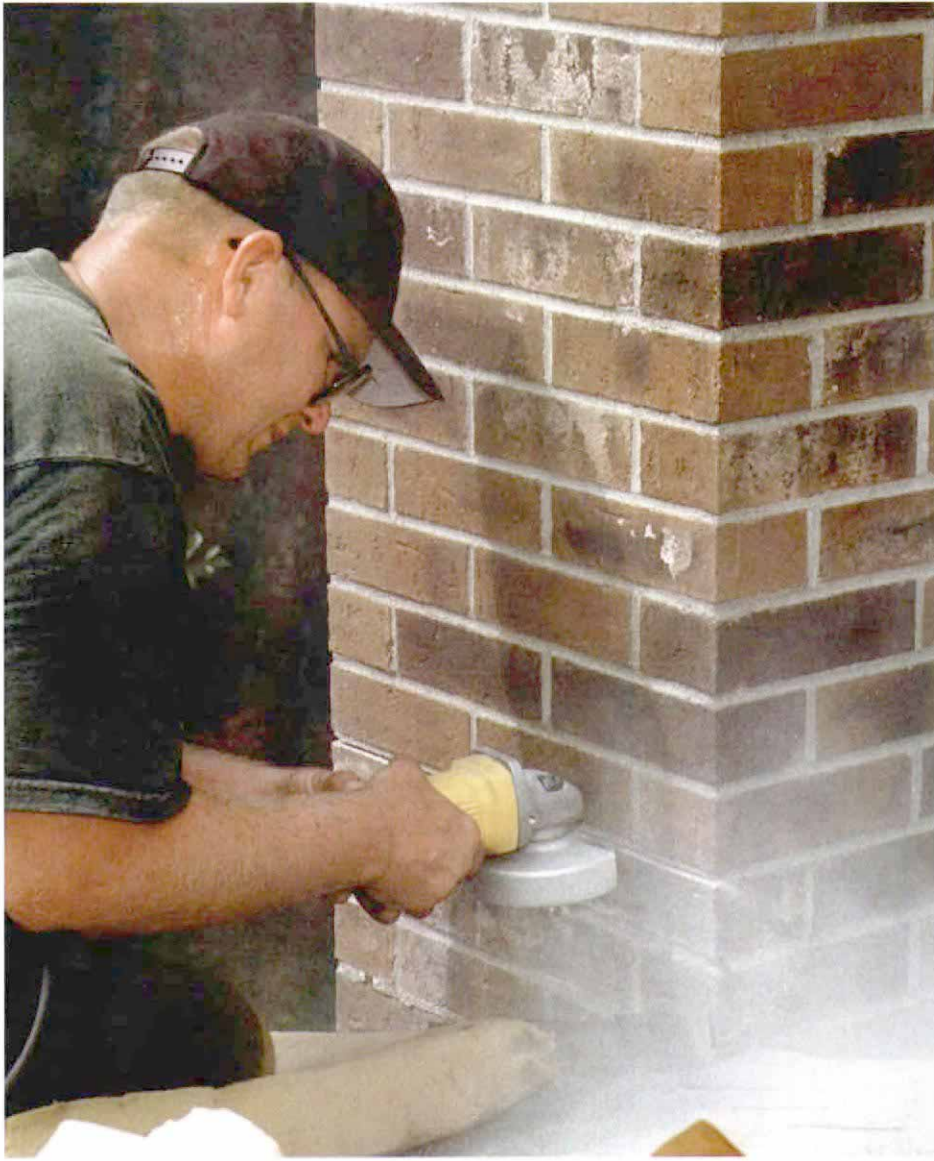
New counterflashing. When reflashing a chimney, the author grinds out the mortar for new counterflashing one course above the old. And yes, he should have used a mask or respirator for this work to protect his lungs.
